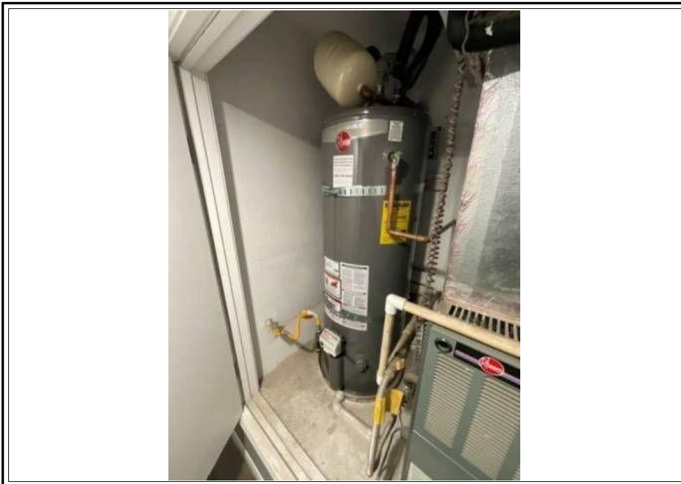
WATER HEATER - DOUBLE STRAPPED
