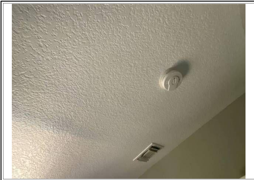
REGISTER SMOKE DETECTOR
