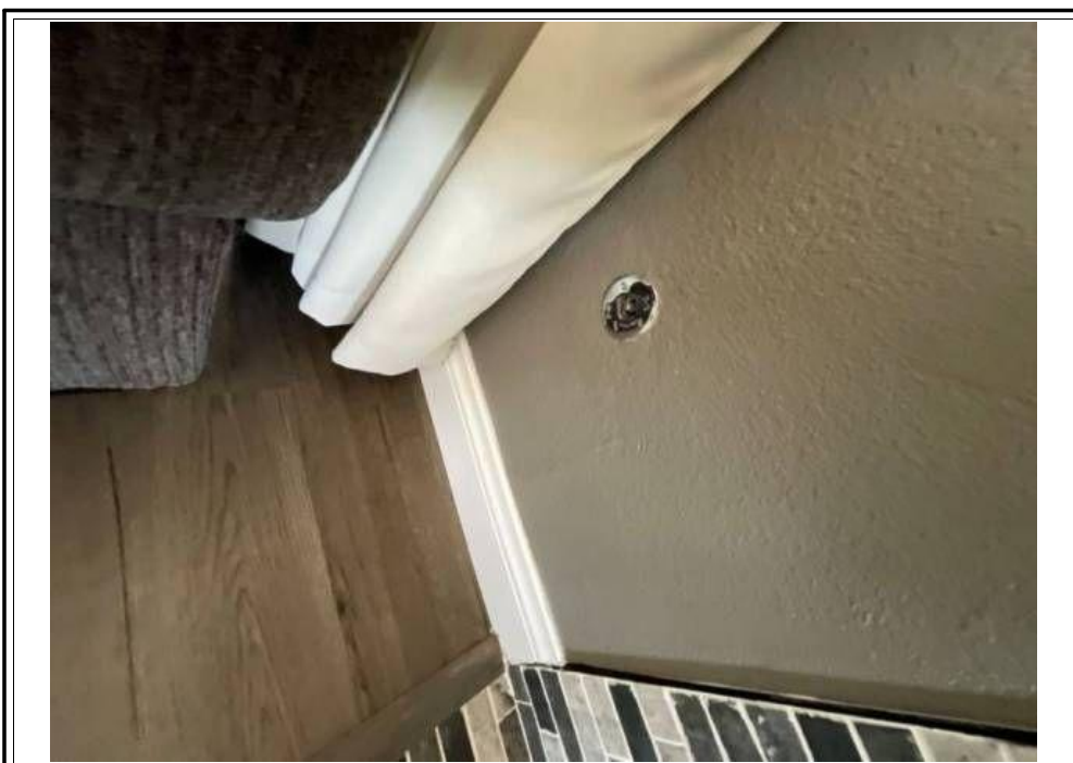
FAMILY ROOM GAS LINE
