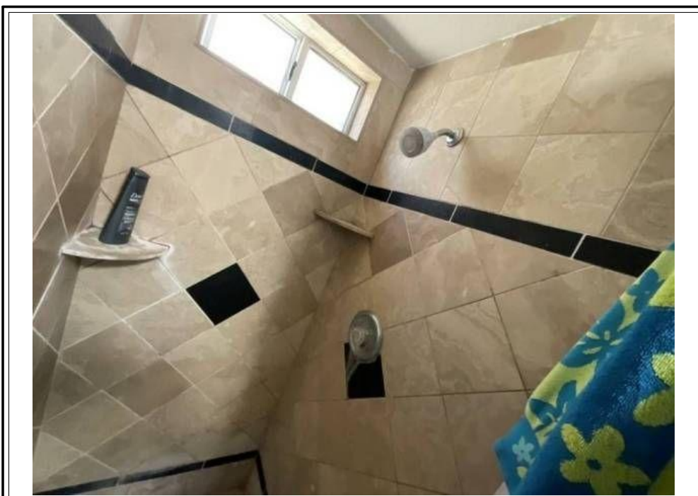
BATHROOM 1 BATHROOM SHOWER HEAD
