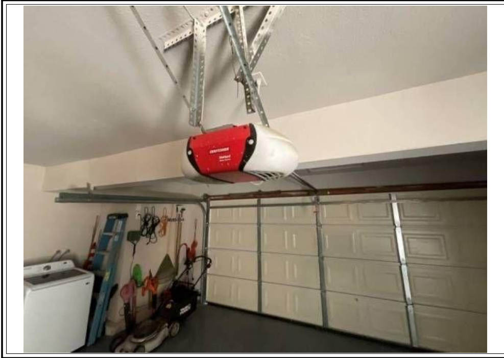
GARAGE AUTOMATIC GARAGE DOOR OPENER
