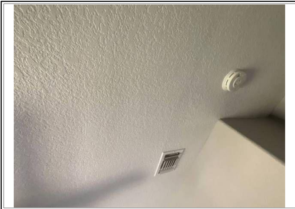
REGISTER SMOKE DETECTOR
