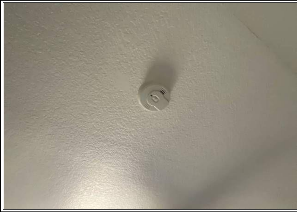
BEDROOM 4 SMOKE DETECTOR
